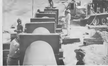
Completing the anchor at a 13-degree bend of the trans-Arabian pipeline, four-and-a-half miles south of Qasimah. The Arab section of the pipeline is a gas pipe line gathering system which ties in with Tapline at Qasimah, in Saudi Arabia.
